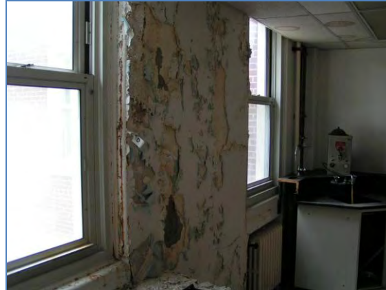
Building 62 also has water damage.
