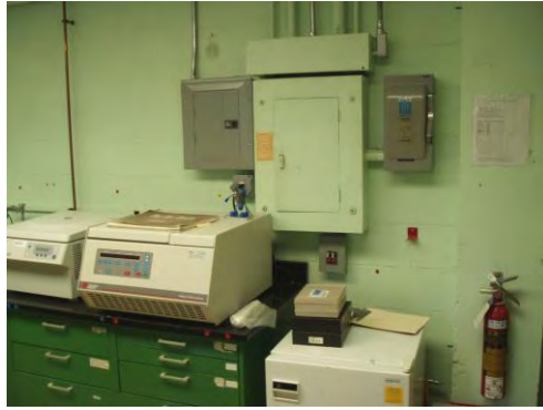
Access to electric panel blocked by equipment in Bldg 44.
