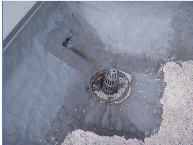
Damaged roof membrane, Bldg 6.
