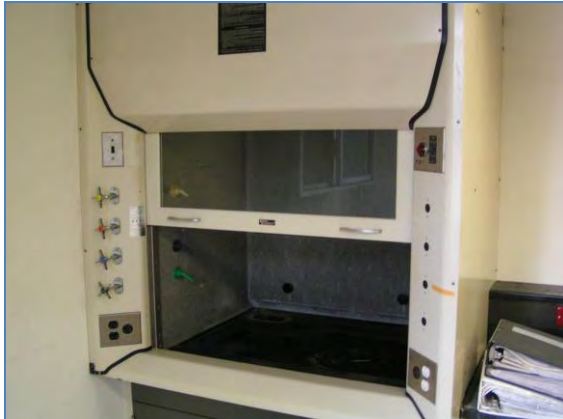
In Building 62, a newer fume hood in a recently renovated laboratory.
