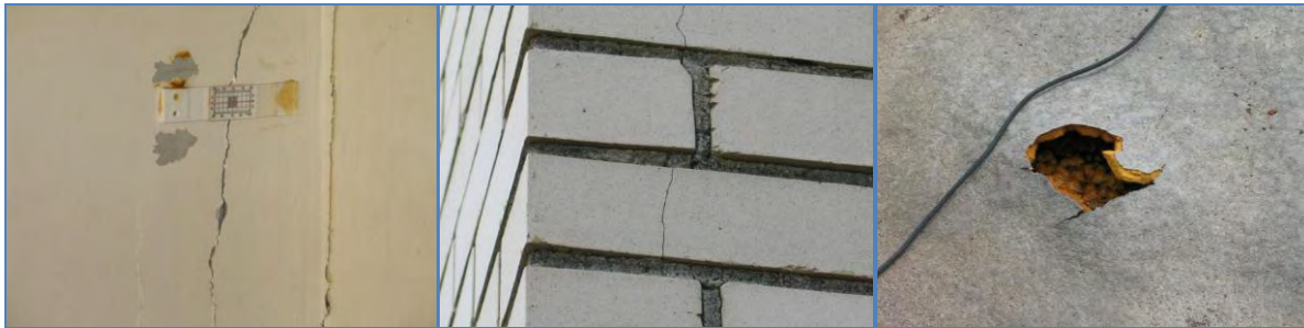
Examples of (left to right): interior cracking, exterior cracking, roof deterioration.
