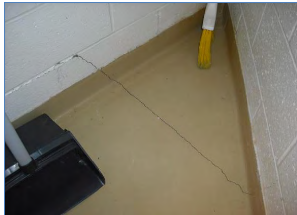
Cracks from the exterior wall across the floor of Building 14.
