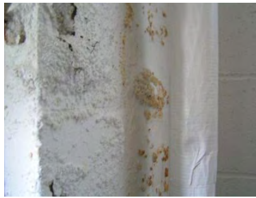
Mold growing in a Bldg 17 laboratory.
