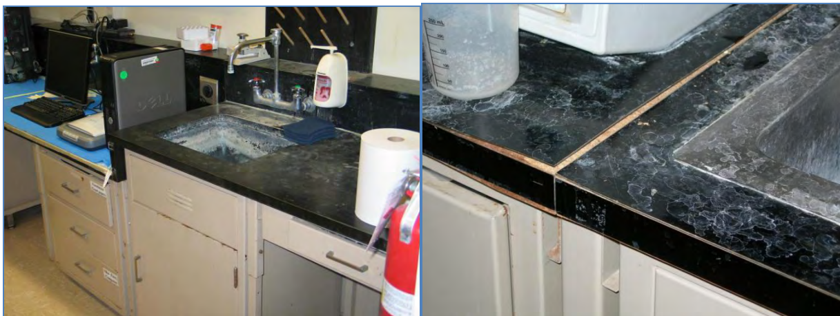
The photo at left depicts typical condition of casework in the laboratories. The photo at right show what can happen when an inappropriate finish (plastic laminate countertop) is used in a laboratory environment.
