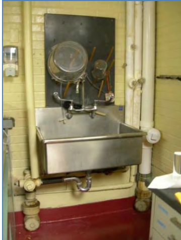
Rusted exposed piping in an animal use area.
