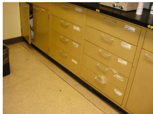
Damaged flooring and rusted casework in Bldg 44.
