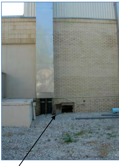
The open hatch at the base of the exterior of Bldg 11 provides a potential inlet for vermin.
