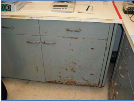
Example of corroded laboratory casework in Building 1.
