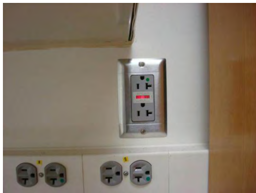
A receptacle protected with transient voltage surge suppression (TVSS).
