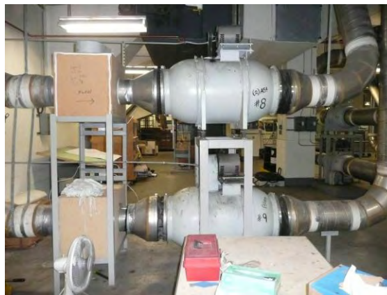
The entire third floor of Building 20 houses mechanical and utility space, protecting equipment from the elements. Shown here are inline fume hood exhaust fans with inlet HEPA cabinets.
