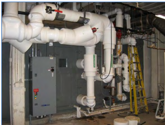
A new air handling unit serving the research space.
