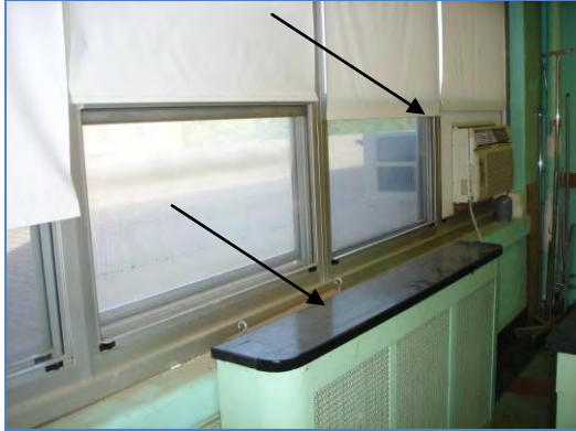
Typical heating and cooling units in laboratories.
