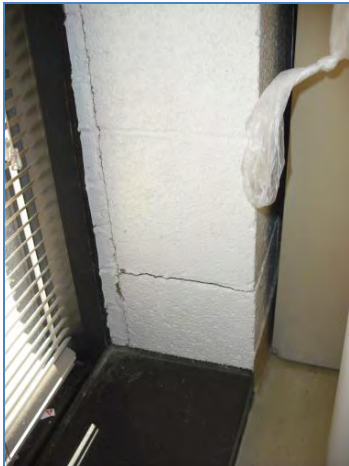
Cracks in exterior wall, Bldg 14.
