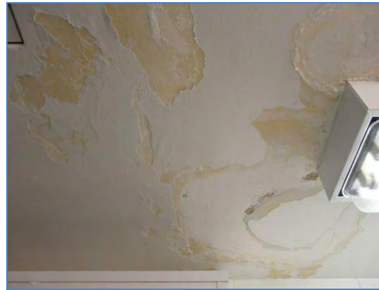
Evidence of leakage in the VMU. A significant leak in May 2010 necessitated evacuation of animals.
