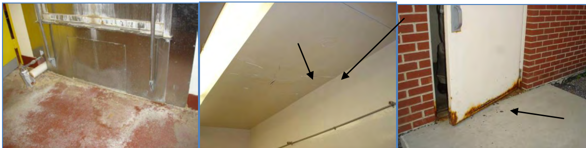
Damaged finishes in the VMU include (left to right) flooring in front of the cage washer, ceilings, and an exterior door.
