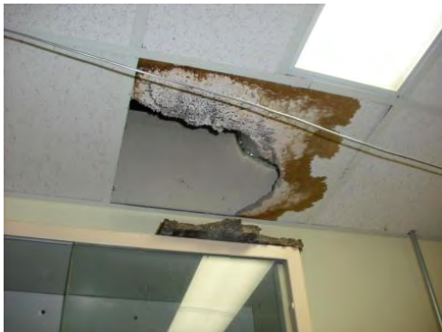
Ceiling damage in Bldg 44.
