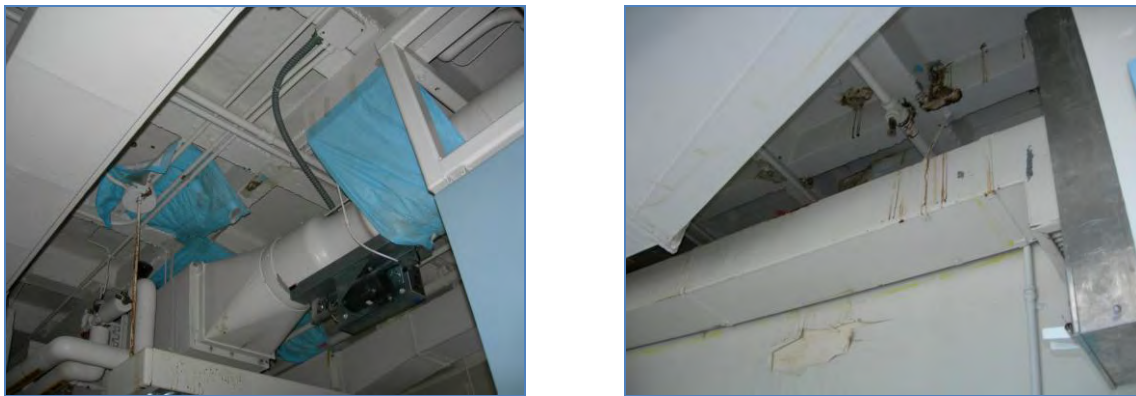
Above, leaks are prevalent in Building 1, due to roof leakage, mechanical equipment, and penetrations.
