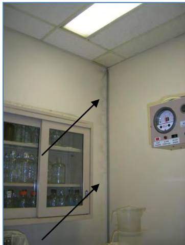
Water damage in a laboratory.
