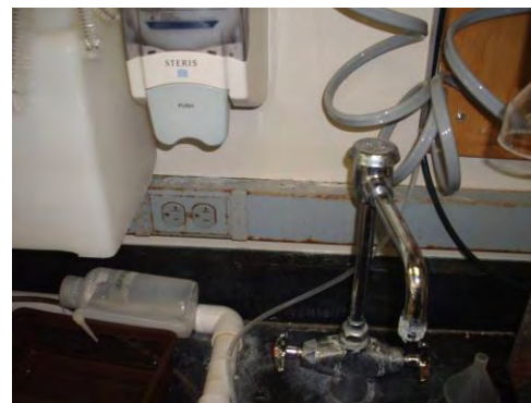
Receptacles near sinks are not ground fault protected. Also note the rusted electrical raceway.
