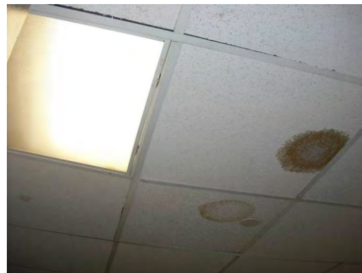
VMU space should have hard ceilings, not acoustic tile. This tile ceiling is damaged. Also note the lack of a gasket on the lighting fixture.
