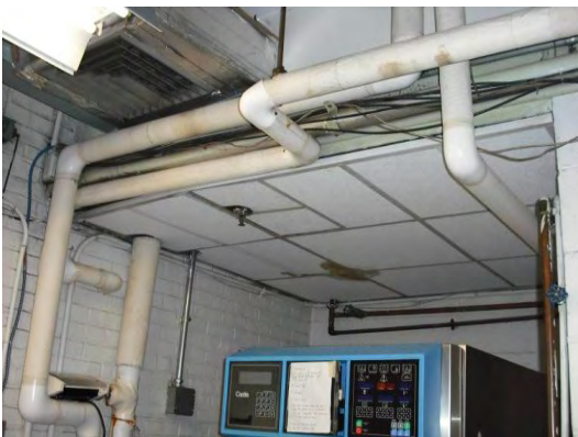
An inappropriate ceiling in the autoclave room, Bldg 20.
