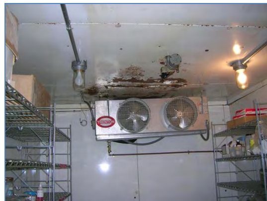
Although this cold room is operational, it has significant physical damage.
