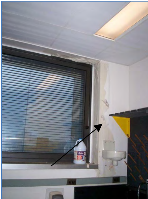
Water leakage around windows has caused significant damage to finishes.
