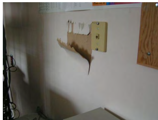
Damage to wall finish caused by water leakage.
