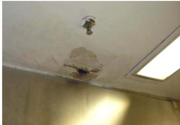
In Bldg 46, damage to an animal holding room ceiling.
