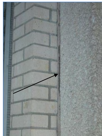
An open joint at the exterior of Building 11.
