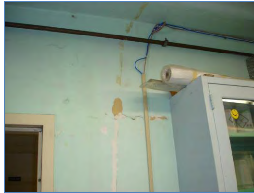
Evidence of water damage is prevalent.
