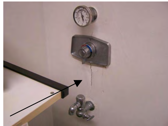
Also in the VMU, this wall behind a faucet has developed cracks.
