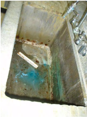
Several laboratories have badly corroded sinks.
