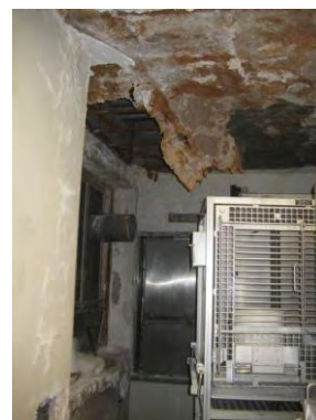
This space on the first floor that has been severely water damaged will be renovated to house freezers.
