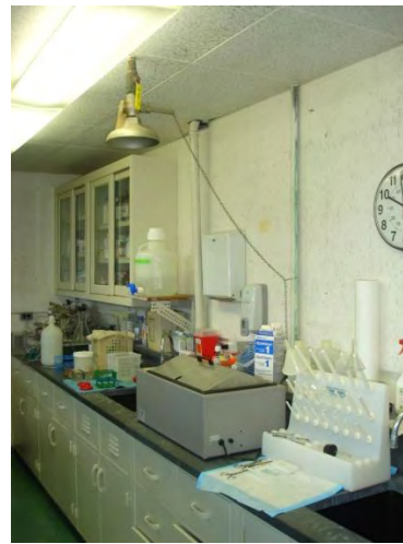
Inaccessible safety shower with equipment requiring electricity below. Safety shower deficiencies have been corrected.
