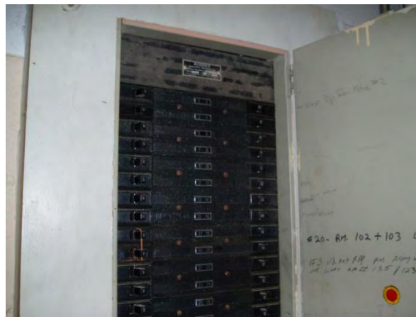
Old style electrical panel in Bldg 46.
