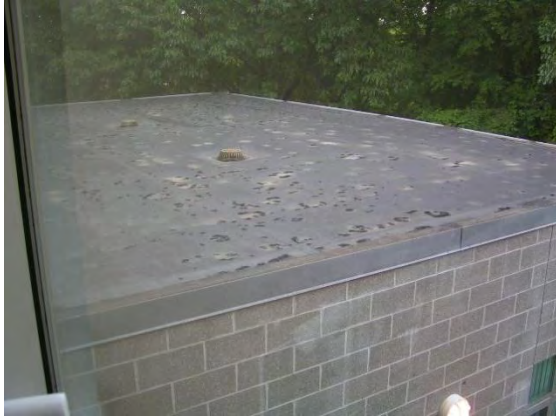
At the time of the assessment, the roof on Bldg 35 had significant leakage.
