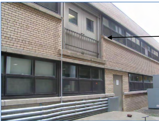
In Building 6 equipment delivered for use on the upper floor must come through this exterior second floor door. There is no elevator in the building.
