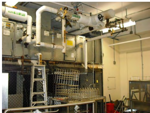
In the VMU, there is no wall between the cage washer and HVAC equipment.
