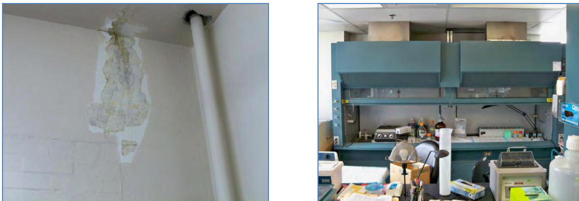
Below (left), Building 8 also has leakage problems causing damage to interior finishes. At right, an aging fume hood in a Building 8 laboratory.
