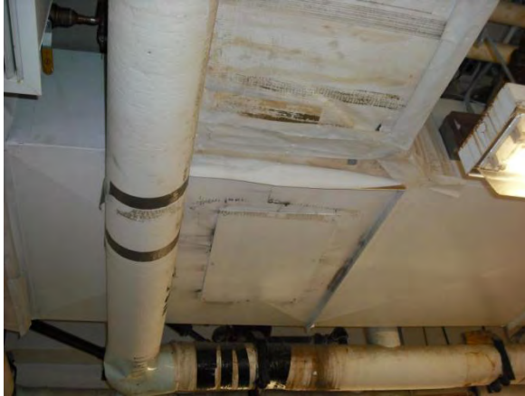
The cage wash area in Bldg 7 has an inappropriate ceiling.
