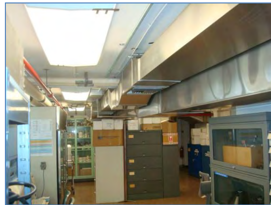
Building 6 has many challenges. This very low exposed ductwork is one of them.
