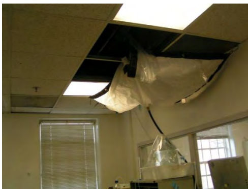
A temporary solution to leakage in a Bldg 70 laboratory. The roof leaks resulting in extensive interior damage.
