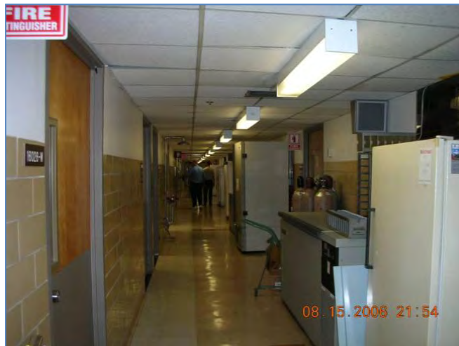
Equipment stored in corridors creates crowded conditions and blocks egress.
